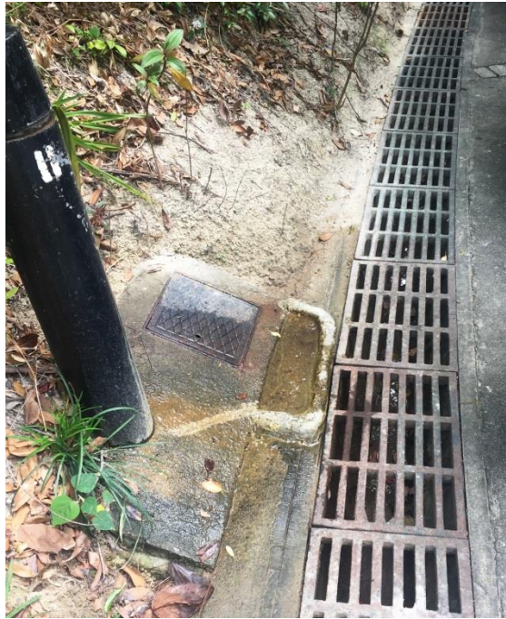
Moistures from leaking pipes often support biting midges infestation
