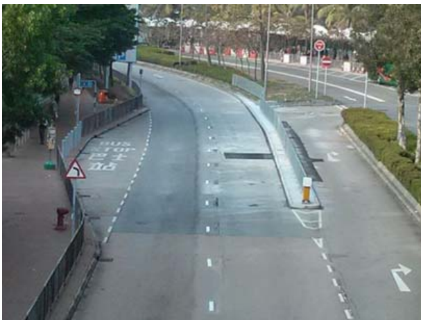
Installing pedestrian railing at central median to prevent pedestrian from crossing the road
