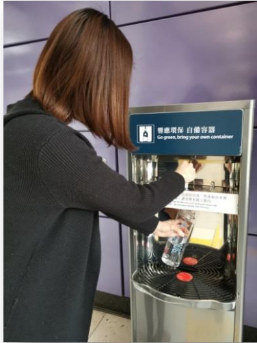
Providing drinking water-dispenser
