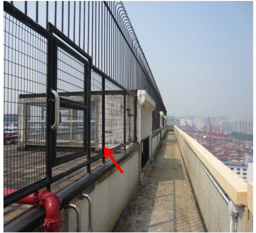
網欄 (建築物屋頂) Mesh fence (on roof)
