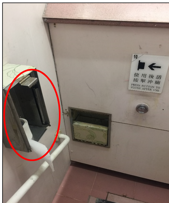
Photograph 4 Defect in toilet paper holder
