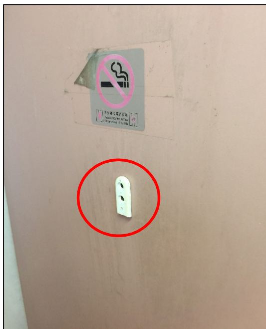
Photograph 3 Defect in coat hook
