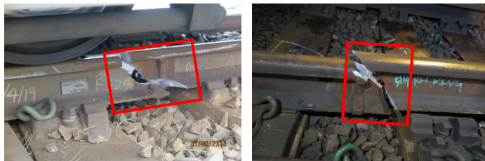
Figure 11 : Two broken rails
