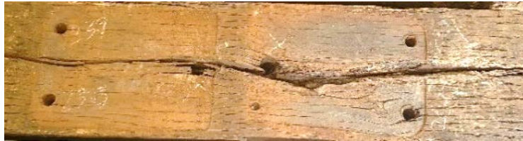
Figure 19 : Rotten timber sleeper
