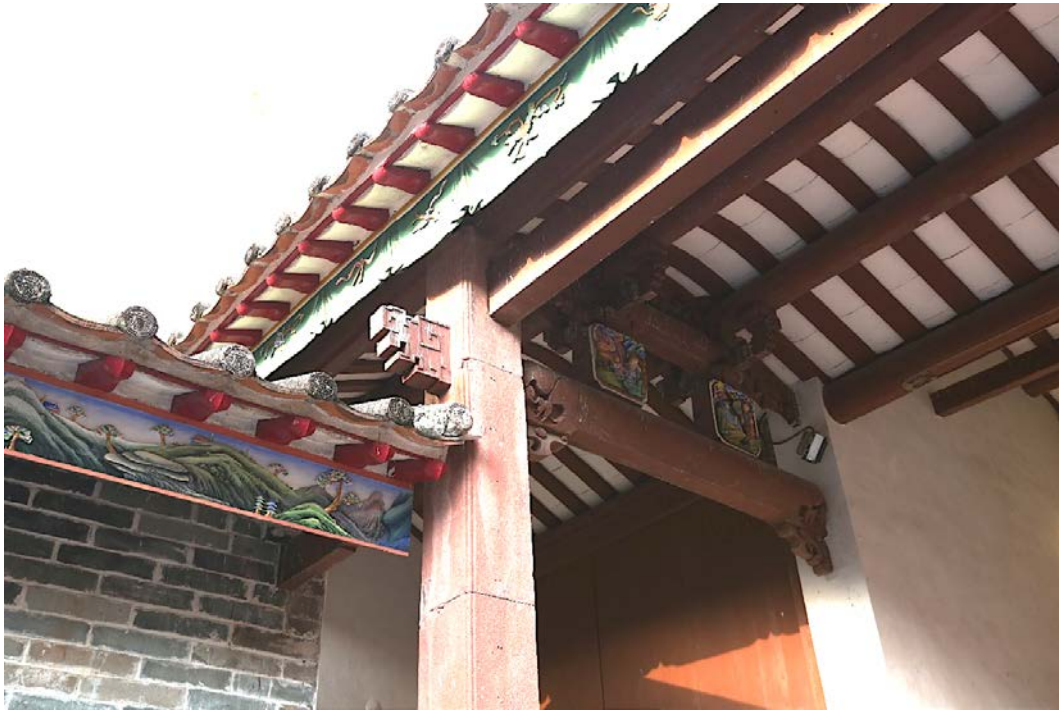
The red sandstone internal eaves column and ornately carved timber beams and camel's humps of the entrance hall
