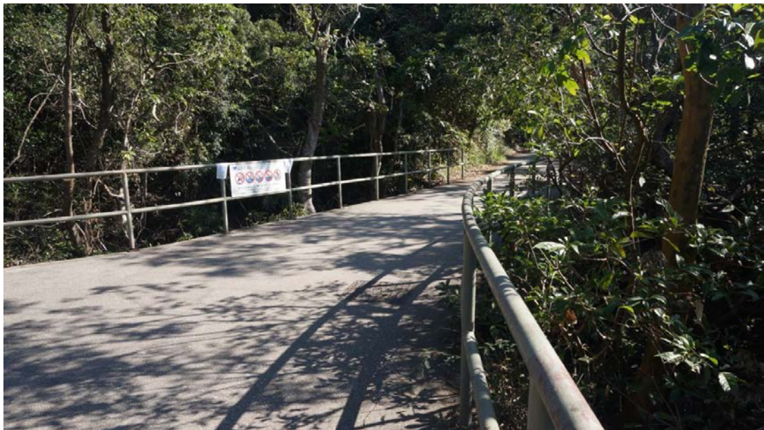
The road surface on top of the Masonry Bridge, which provides indispensable linkage with other waterworks facilities of Pok Fu Lam Reservoir.
