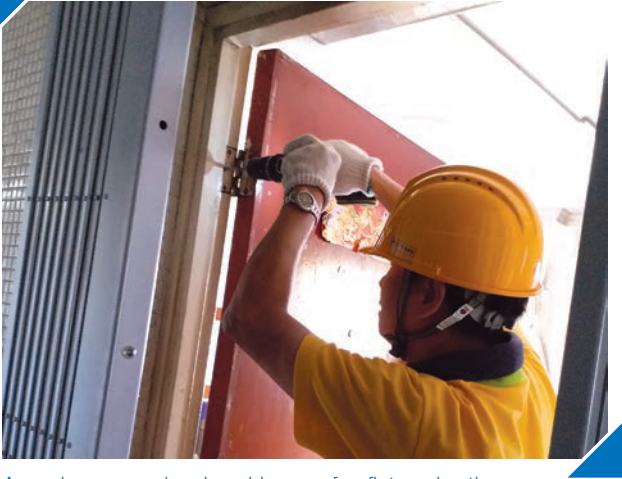
A workman repairs door hinges of a flat under the Responsive In-flat Maintenance Services
