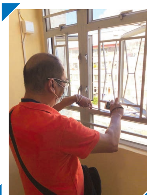
A “Qualified Person” undertaking a mandatory window inspection at Lai Kok Estate
