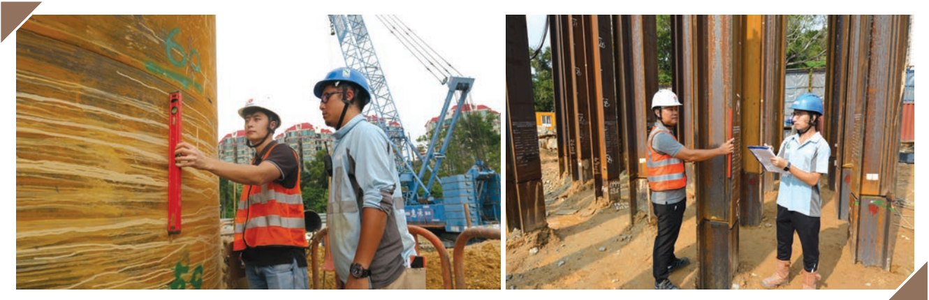
Measuring the verticality of pile steel casing (left) and supervising the construction of driven H-piles to ensure building quality
