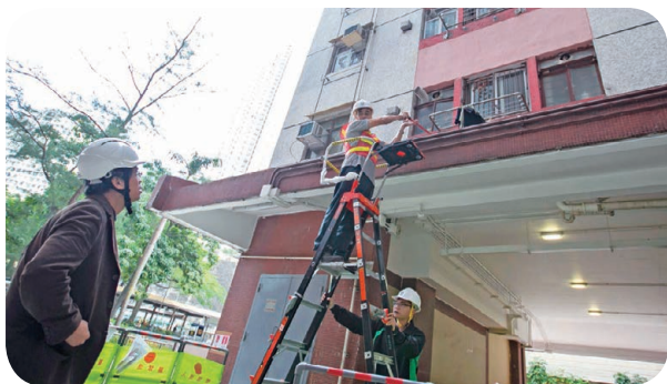
物業管理公司委託本局，進行安全稽核，我們在過程中提出改善職安健的建議。 We were commissioned by property management companies to conduct safety audit and made recommendations to improve OSH performance.
