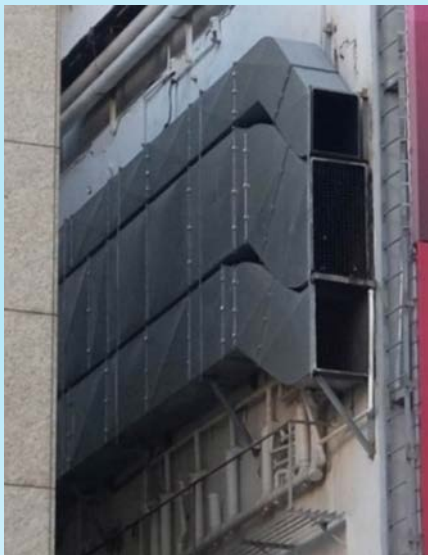
金屬通風管道或任何相關的承托支架 Metal ventilation duct or any associated supporting frame
