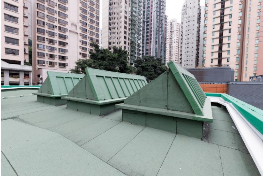
The three skylights on the roof have been blocked
