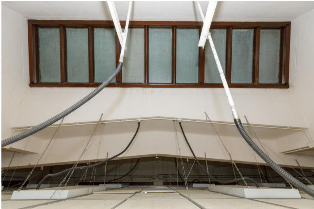
Pitched beams and the undersides of the blocked skylights made up of timber frames and glass panes could be found above the false ceiling in the Art Room on the second floor
