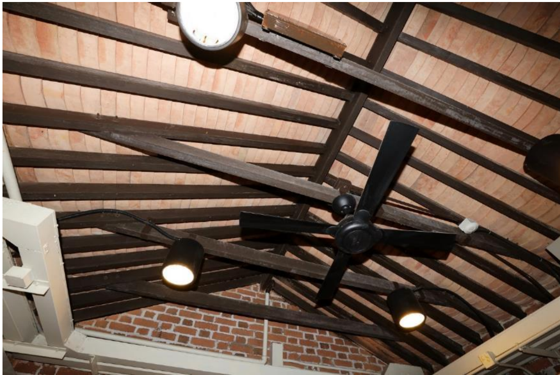
Chinese styled tiled pitched roofs supported by timber battens and purlins at Staff Quarters Block
