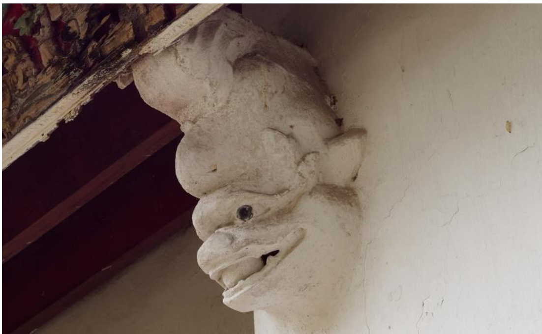
One of the two corbels plastered in the shape of dragonfish supporting the façade eaves
