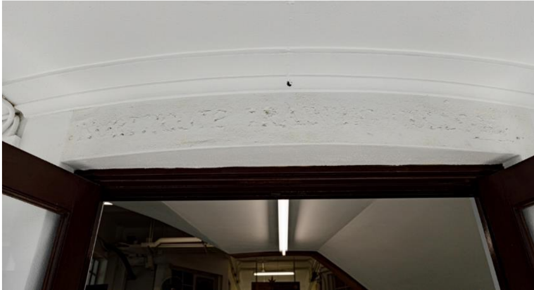
The trace of the name “Northcote Training College” at the main entrance on the south elevation of the main building
