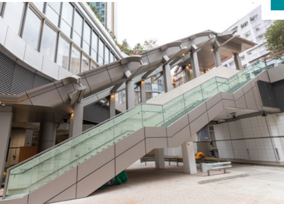
The Air Induction Units installed at the Yue Man Square Public Transport Interchange help improve the airflow with less energy consumption.
