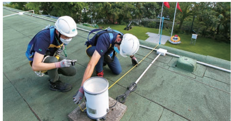
顧問團隊為設於屋頂上的自動氣象站進行實地測量，以評估天文台員工於該處工作時可能面對的風險。 The consultant team took site measurements for the automatic weather station located on the roof to assess the potential hazards that the observatory staff might face while working at the site.
