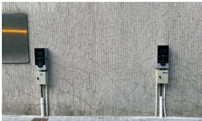
Electric Vehicle charging facilities in the car park. 停車場電動車充電設施。
