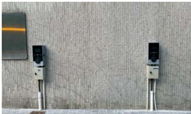
Electric Vehicle charging facilities in the car park. 停車場電動車充電設施。
