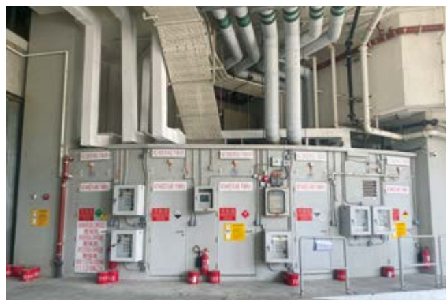
The new Dangerous Goods Store in the Theatre Block. 新危險倉庫設於劇院大樓地下高層。
